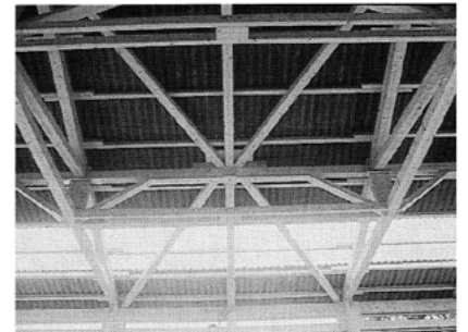
Girder in the plane of the roof for bracing and providing restraint to the top chord of the roof truss, purlin frame for providing restraint to the bottom chord against uplift wind forces
