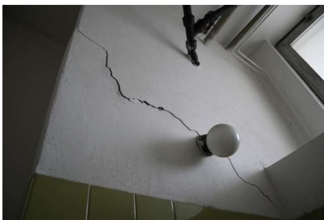
Fig.176 0-31, trhľina v stene
